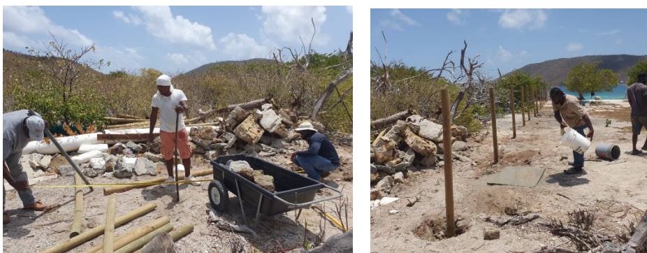
Above: NPTVI Staff installs fence at Prickly Pear National Park, Prickly Pear Island (North Sound, Virgin Gorda)
